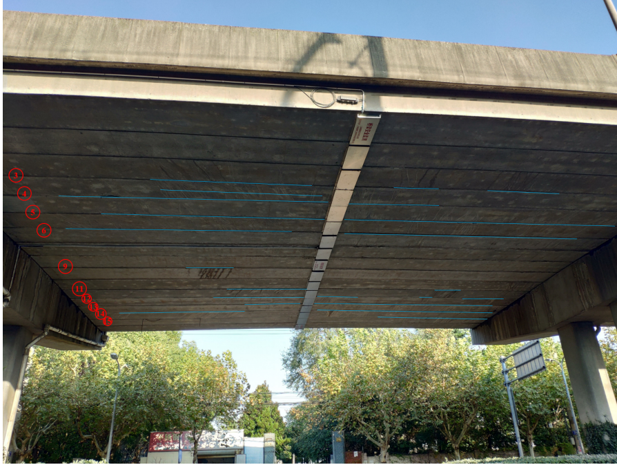
Fig. 19. Field picture of K92 on November 23, 2018. The blue line denotes locations of damaged hinge joints causing evident water leakage.
