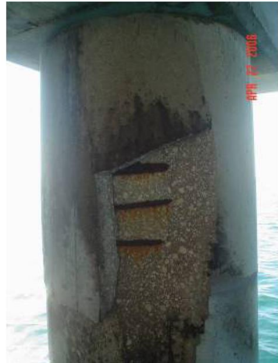
Figure 4: Extensive corrosion damage[3]
