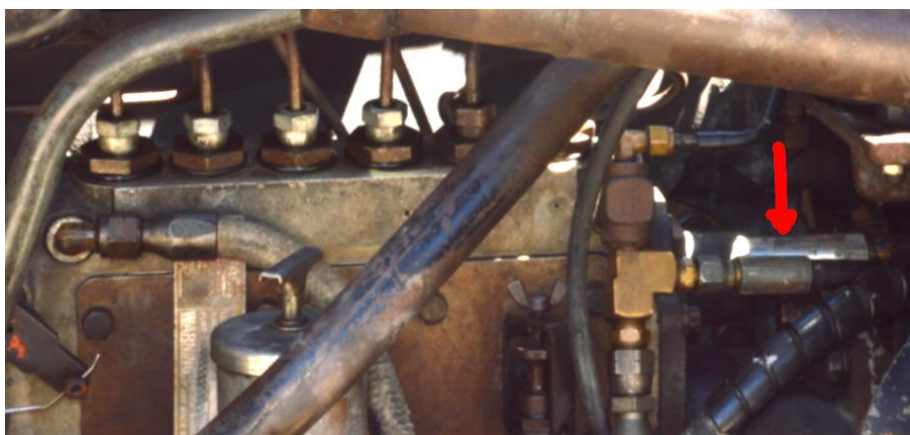
Figure 29 - Puff control device highlighted by red arrow.
