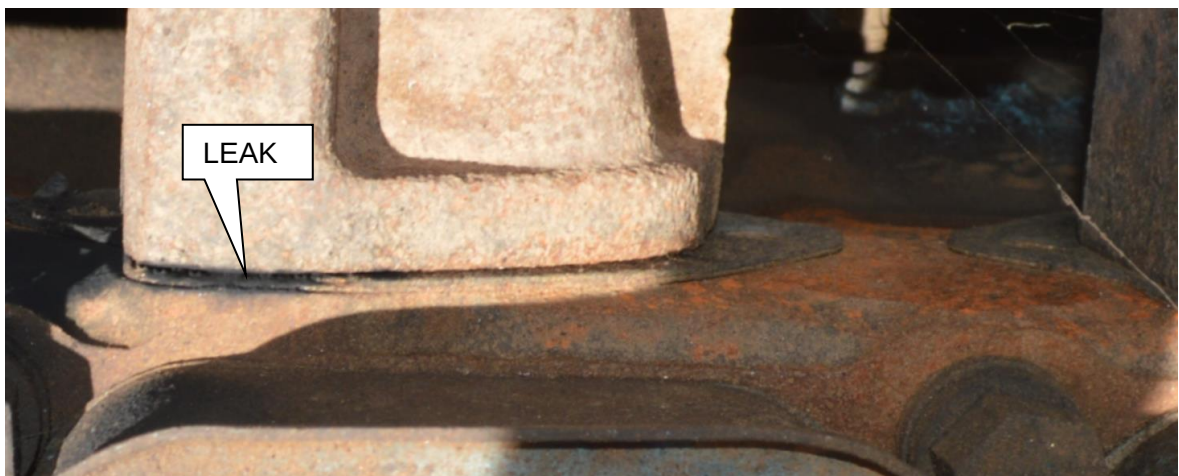
Figure 9 – Photo taken by the author highlighting exhaust gas leakage.
