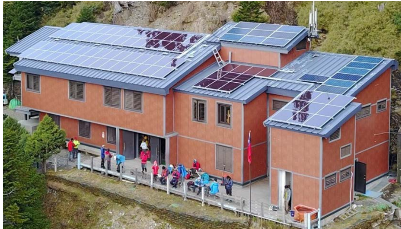
Solar Energy storage system (system integration)
