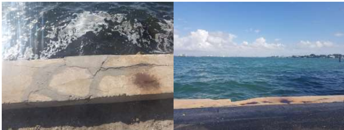
Figure 2: Seawalls showing evident corrosion damage.
