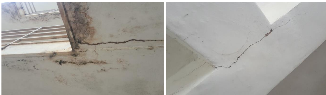
Fig. 2 Cracks on structural beam and slab: classroom and dormitory, Woliso Campus
