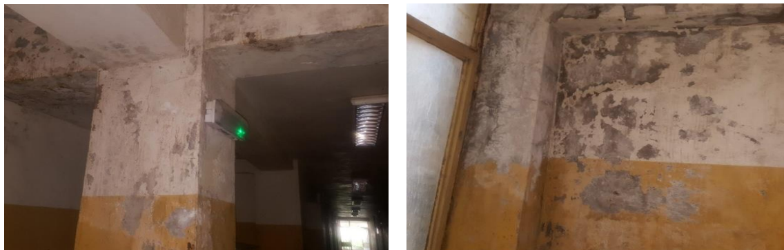
Fig. 3 Moisture leakage problems: dormitory blocks, main Campus
