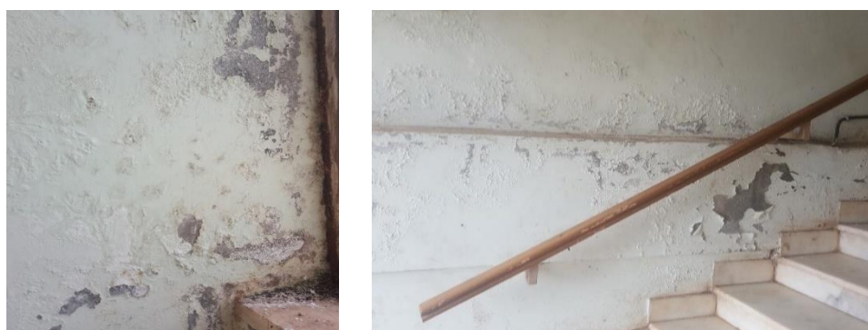
Fig. 4 Paint defects observed on walls from the four campuses.
