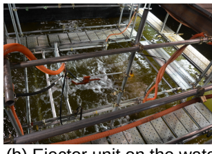
(b) Ejector unit on the water surface
