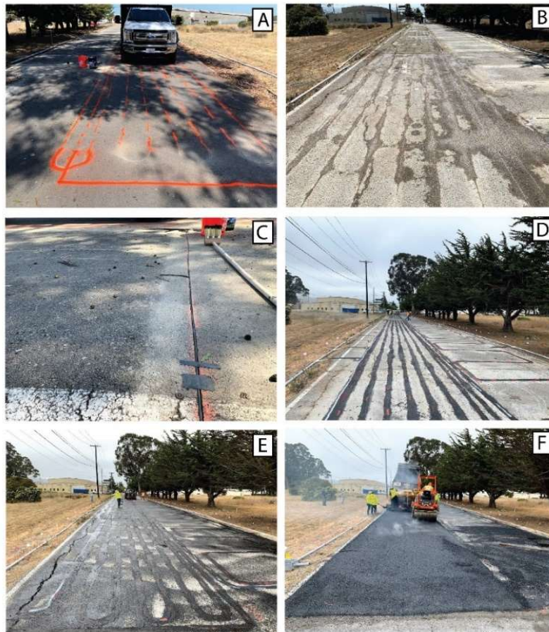
Figure 3. The fiber optic sensing cable installation procedure consisted of (a) marking the locations of the cables on the existing road surface with marking paint, (b) cutting grooves into the pavement surface 5 mm deep with a pavement saw, (c) laying the NZS-DSS-C02 sensing cable into the grooves and securing temporarily with tape, (d) applying a mixture of asphalt emulsion and sand to the top of the grooves to protect the cables, (e) applying a tack coat to the entire road surface and (f) paving the surface using the standard procedure including placing the HMA with a paving machine and vibro-compacting it.
