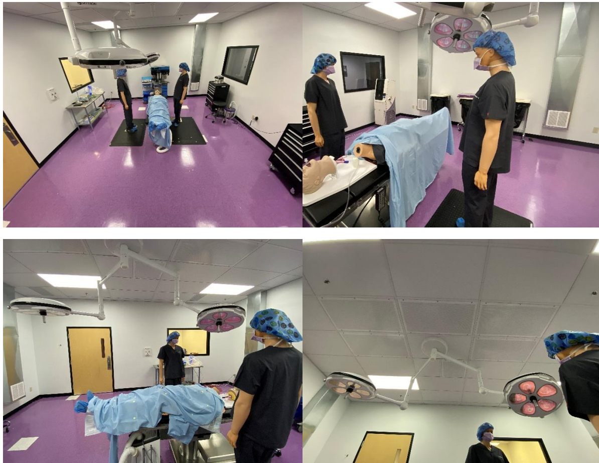
Figure 1: The configuration of the simulated operating room during airflow measurements is shown. The position of the Illuvia Sense is shown in the upper right image. The ceiling mounted vents are shown in the lower right image.
