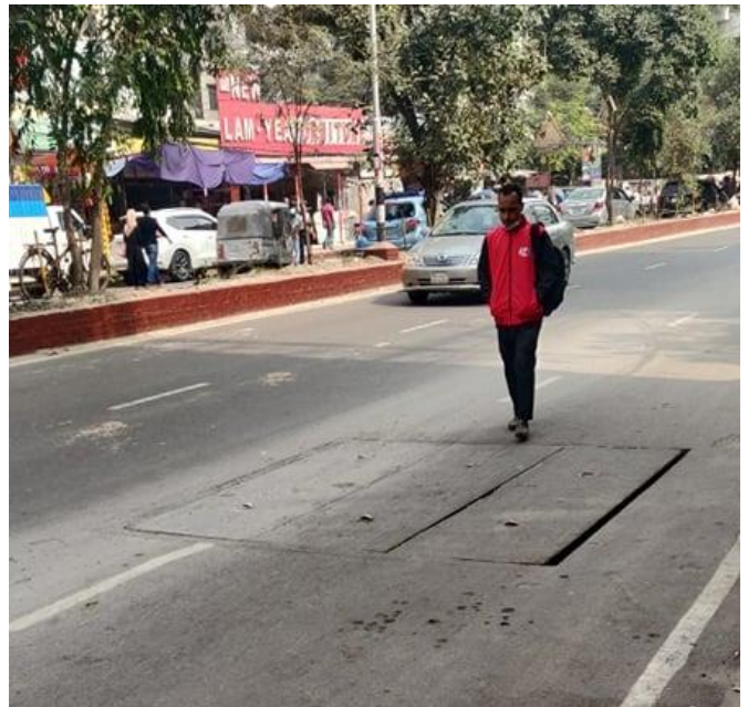
Figure 16: Unhinged Utility Hatches
