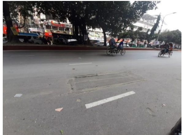
Figure 14: Depressed Utility Hatch
