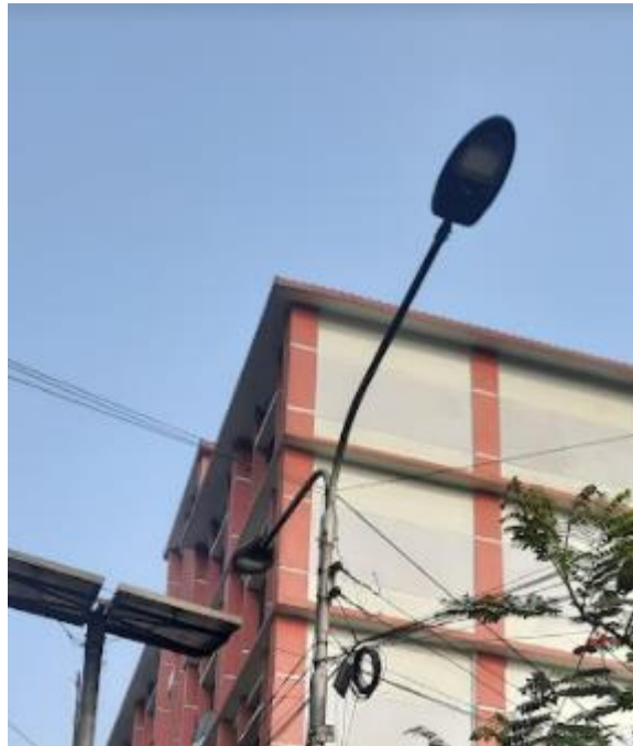
Figure 37: Street Lights in the Corridor
