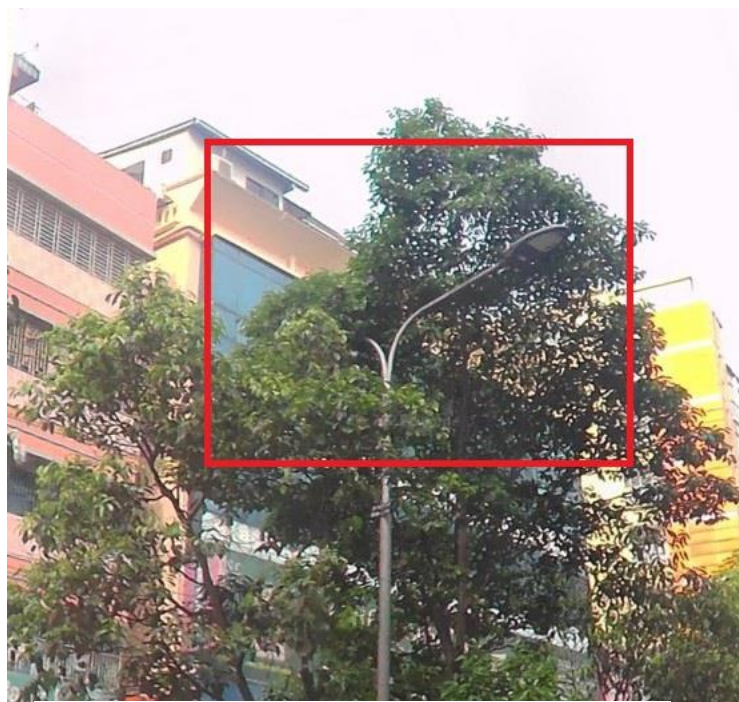
Figure 37: Street Lights Obstructed by Tree
