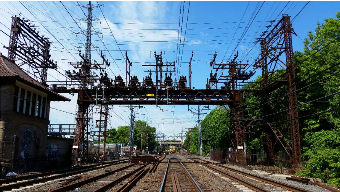
Figure 9. Passenger Railway Supply Substation on the Northeast Corridor.
