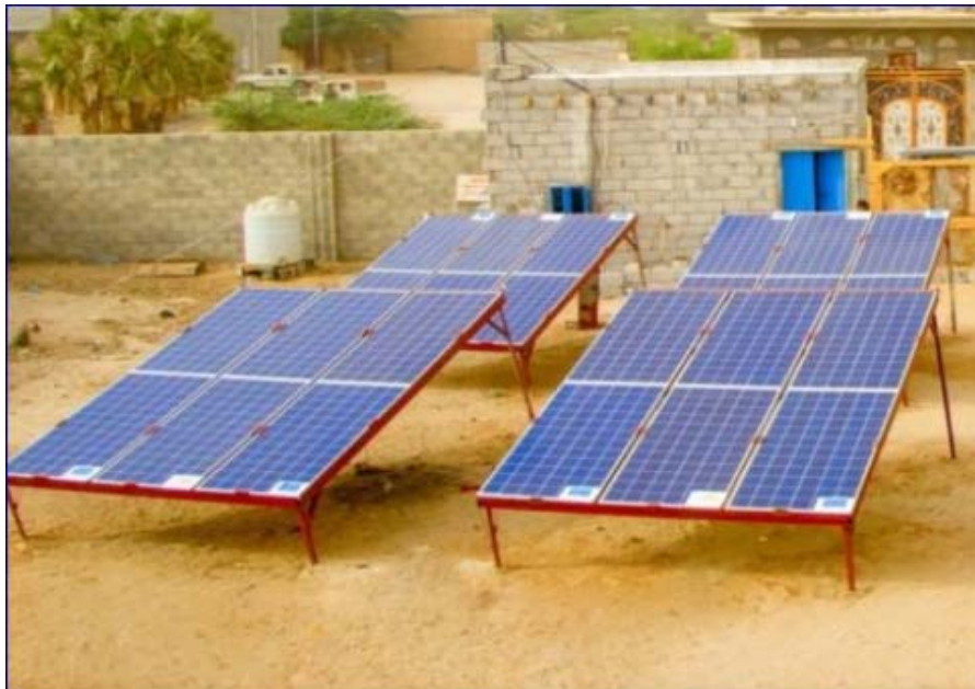
Figure 9. Show atypical Solar energy for Rural Areas Electrification ( Simple Microgrid)[32]
