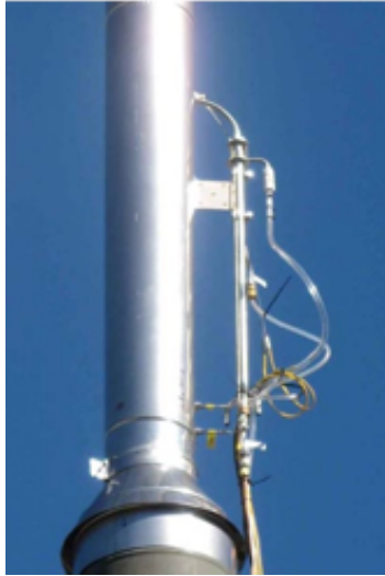
Figure 5. Flue extension and venturi diluter mounted to the outlet of wood heater chimney [44].
