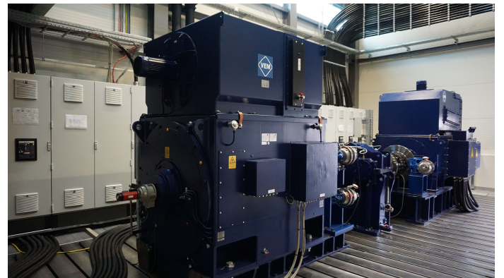
Fig. 4. Large generator Lab; DFIG and PMSM wind generators
