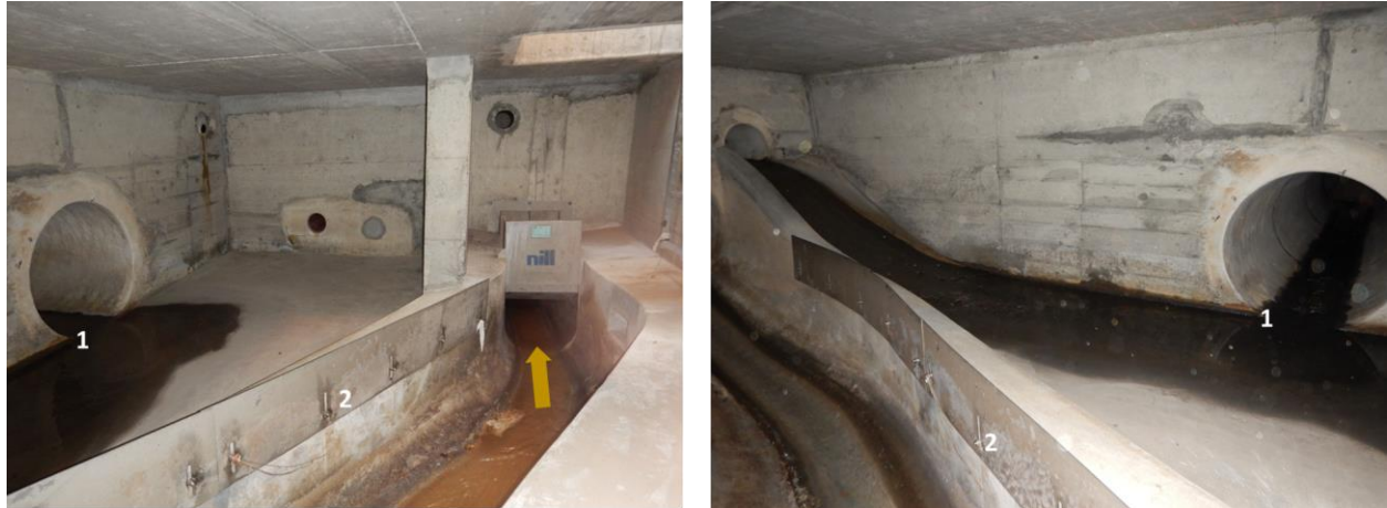
Figure S 3-9: Overflow chamber RU 40a with slide gates (photos taken from HBT, 2016; modified). The left and right pictures show a downstream and upstream view. The numbers 1 and 2 label same points of reference and the arrow indicates downstream flow direction.
