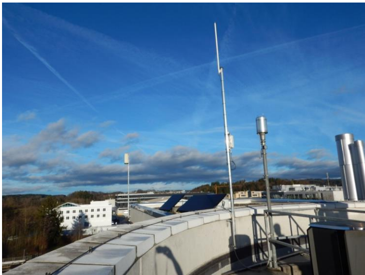
Figure S 4-16: Gateway at the rooftop of the Fehraltorf WWTP control building.
