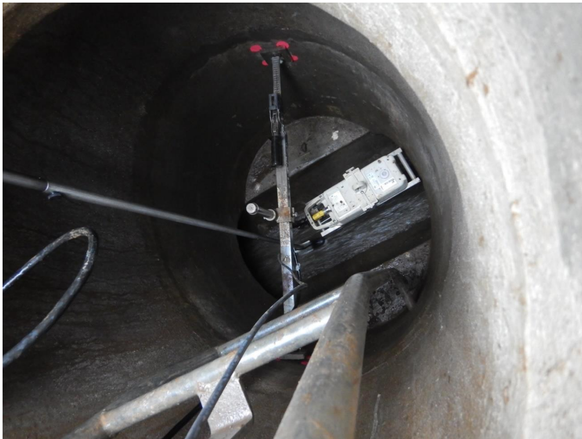
Figure S 4-6: Flo-Dar installed in manhole during comparison with portable flow meter
