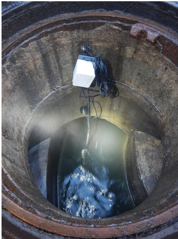
Figure S 4-5 Example installation of a dual temperature sensor, which simultaneously record temperatures of the wastewater and the sewer atmosphere.
