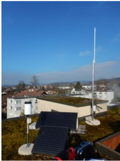
Figure S 4-15: Gateway at the rooftop of a high rise building, including solar panels powering the entire system.
