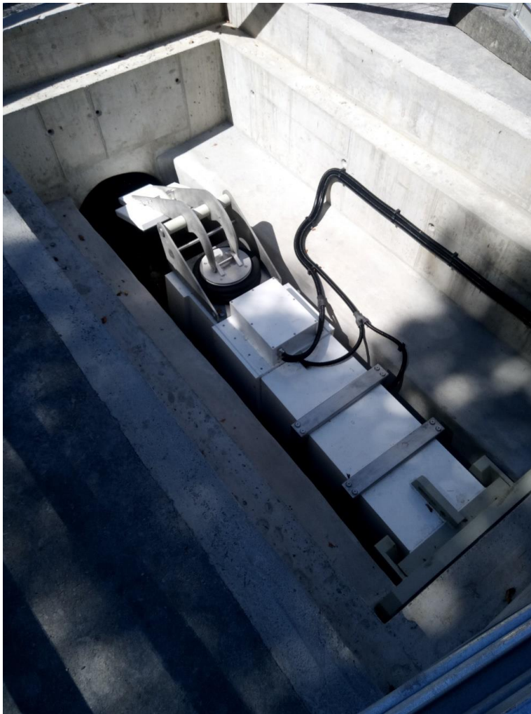
Figure S 4-12: pneumatic flow limiter, partially-filled, at the main collector just upstream of the WWTP inlet.
