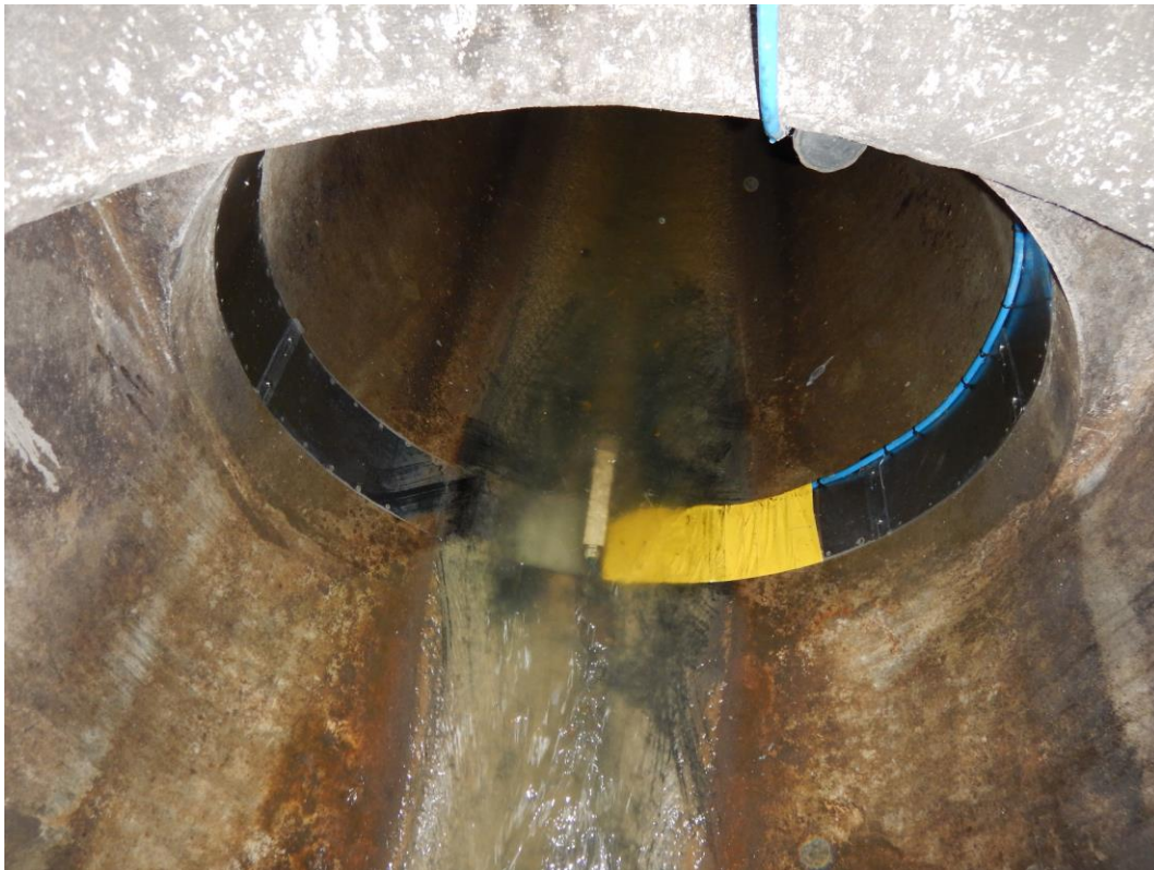
Figure S 4-8: Nivus POA correlation wedge sensor(barely seen on the ground) inside the sewer
