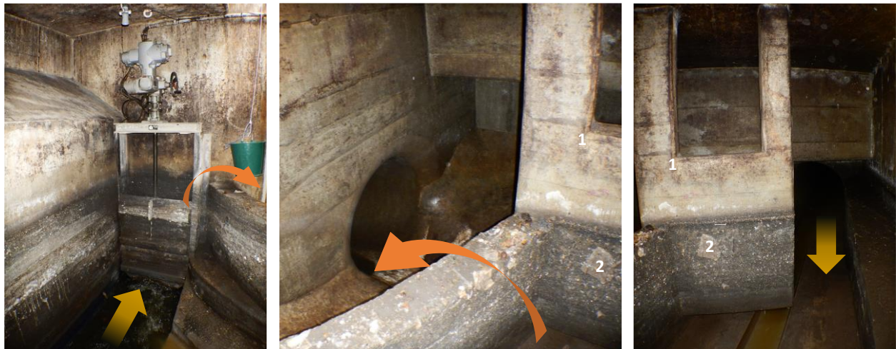
Figure S 3-10: In-sewer flow diversion structure US 58 . Until mid-2020, the penstock actuator served as the primary control element to limit the inflow to the WWTP. The bottom channel (left picture) is the main dry weather inflow towards the WWTP. Middle picture: broad-crested overflow weir and inlet into the in-sewer storage channel that runs in parallel towards the RUB 59 (RUB ARA) .
