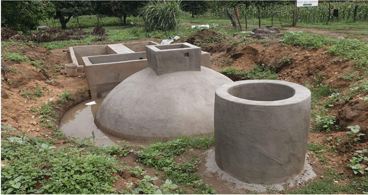
Figure 7.6: Fixed cover digester in work.
