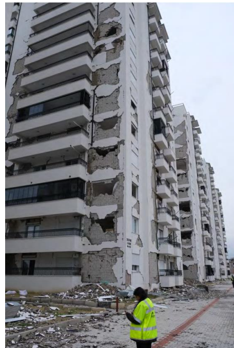
(b) In-plane and out-of-plane damages [9]
