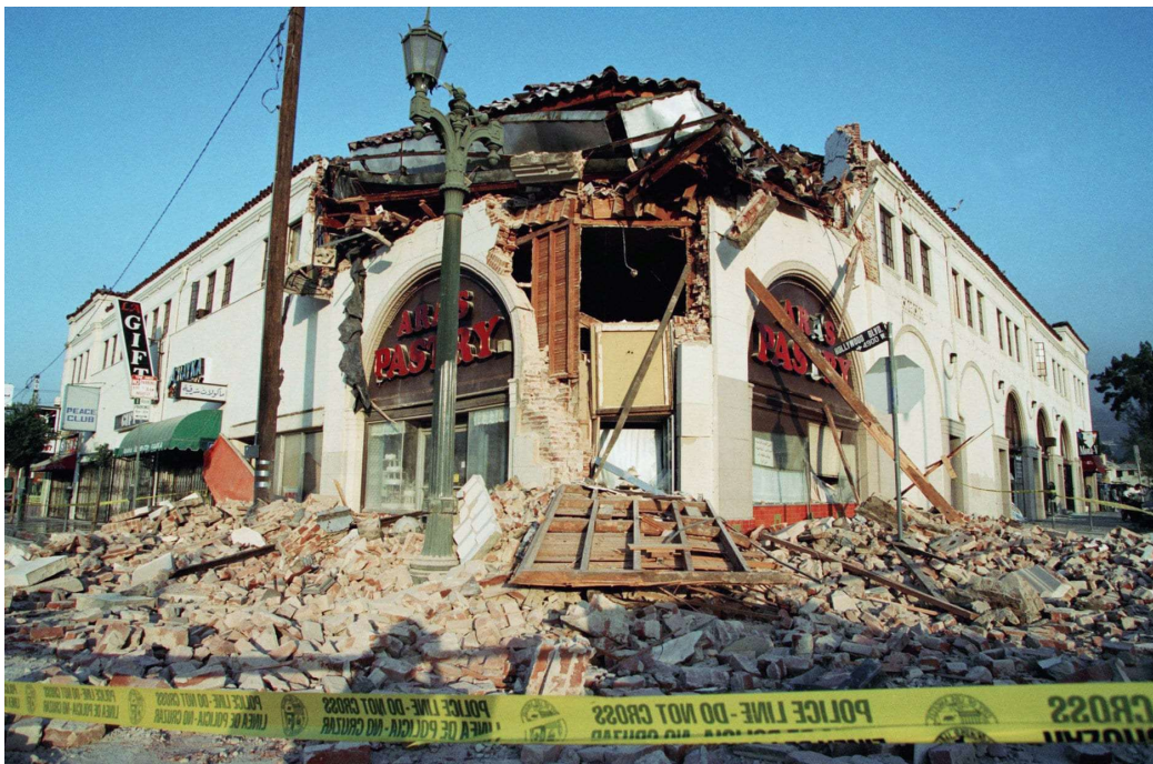
Figure 3:Northridge Earthquake, USA (1994)
