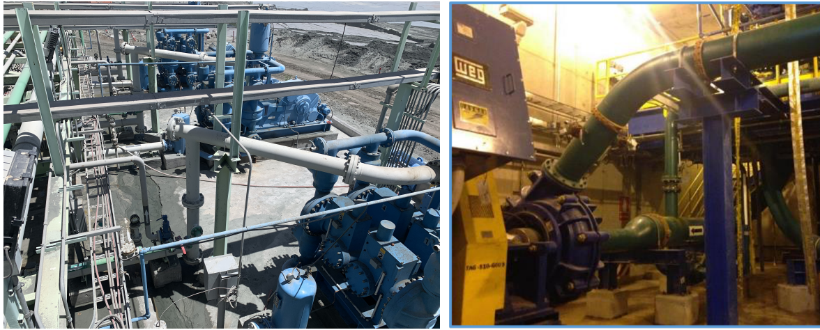
(a) Piston-diaphragm slurry positive displacement (PD) pump (blue equipment)
