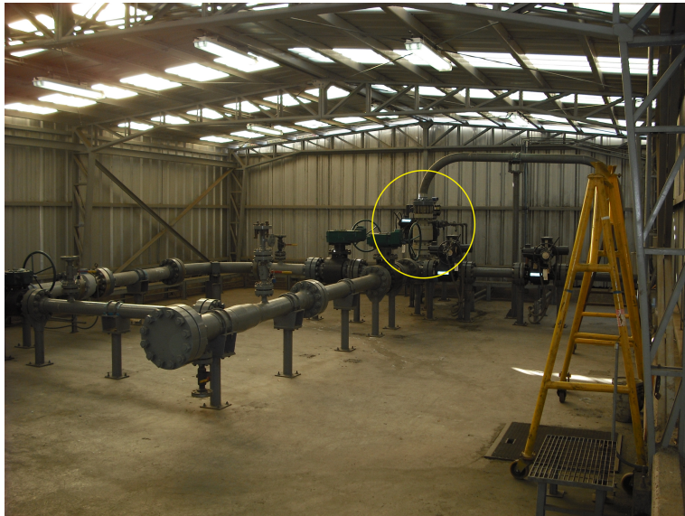
(b) Rupture disk (circled) on the upstream side
