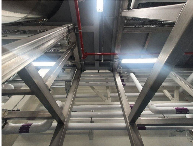
Figure 3 Stainless steel maintenance platform in a 'clean room' in a biopharmaceutical product plant.
