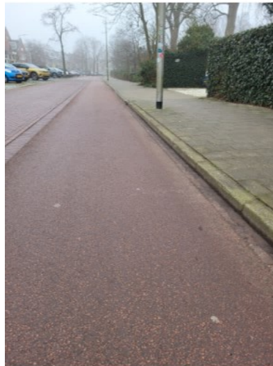
Figure 22: Tarmac test area. ALT TEXT: Photo of tarmac for strollers.
