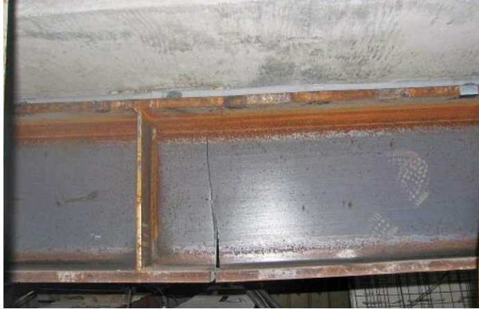
Figure 2. Fatigue fracture failure of composite beam [29]
