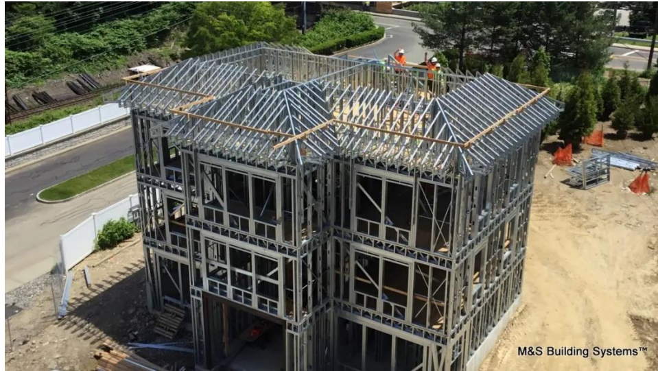
Figure 3. Cold-formed steel truss system in a multi-story commercial building, showcasing the lightweight and efficient structural framework.
