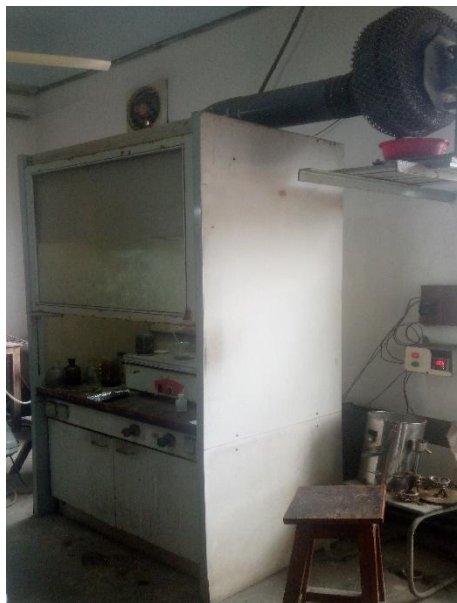
Figure 24: reaction under exhaust fan
