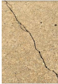
259 Fig. 12: Concrete Crack
