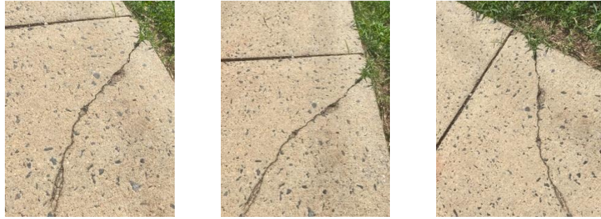
Fig. 1.1: Sample crack images acquired under slight viewpoint variations.
