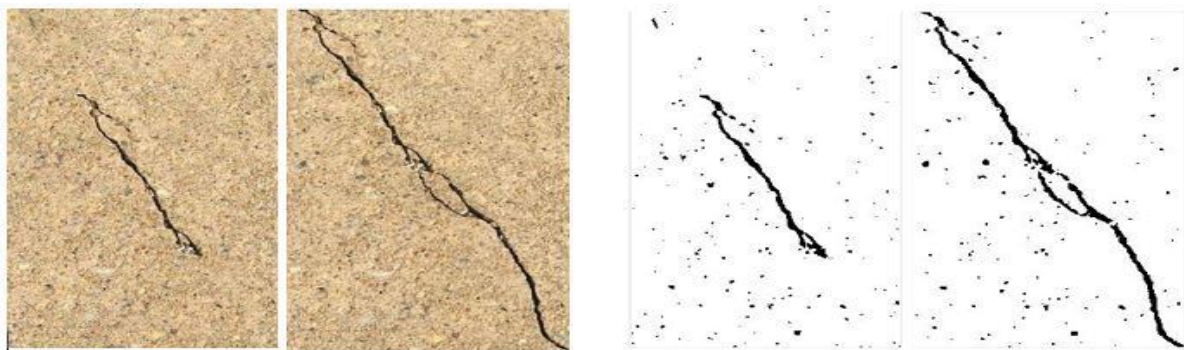
Original crack images
