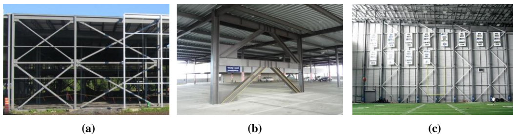
Figure 1- The various configurations of multi-tier braced frames (a) multi-tiered concentrically braced frames (MT-CBF) (b) multi-tiered eccentrically braced frames (MT-EBF) (c) multi-tiered buckling-restrained braced frames (MT-BRBF) [5]
