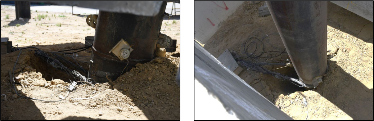
(a) Near Ground Go-Pro Photo Looking West (b) Looking from above the Concrete Blocks
