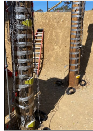
c) In-ground DC Accelerometers
