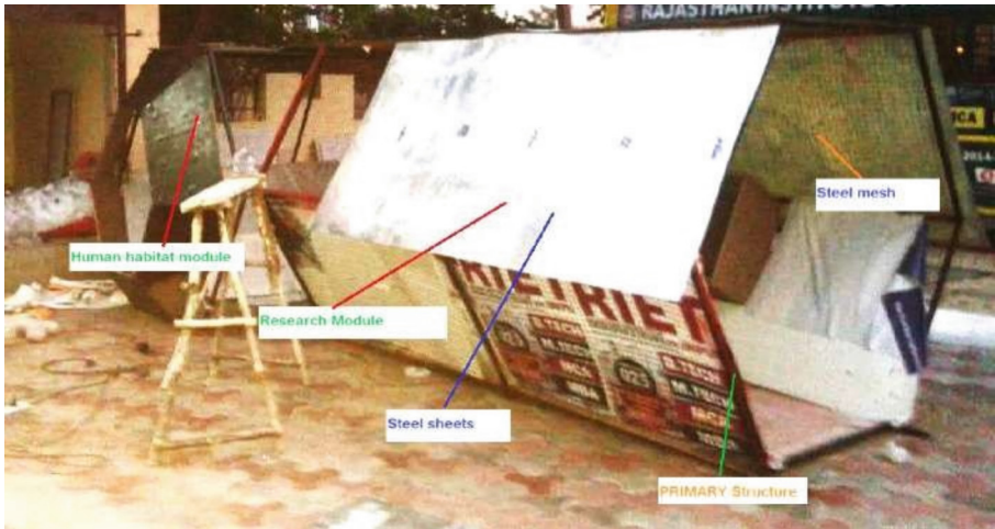
Fig. 16. Primary structure and secondary support structure of research section under construction – module 1729
