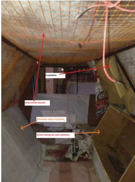
Fig. 17. Primary structure and secondary support structure with sub-system casing, insulation, finishing material during construction – module 1729
