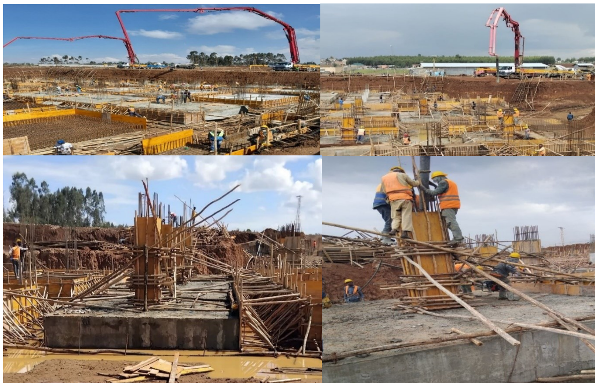
Figure 2.15 Placement of Concrete for Footing Pads and Column Starters via Pump Truck.
