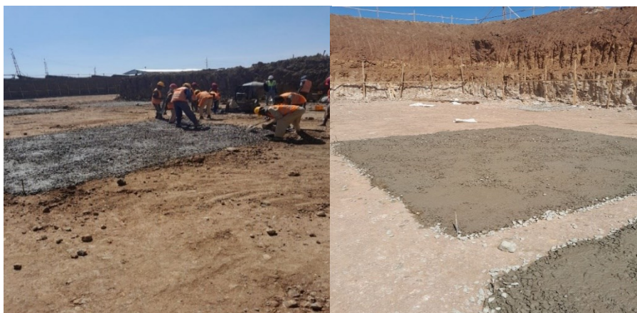
Figure 2.12 Lean Concrete Mixing using a Drum Batch Mixer and Placement under MHB Footings.
