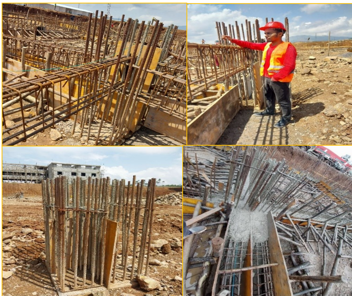
Figure 2.25 Expansion Joint Construction Layout on Site, at basement Columns and Beams of MHB.
