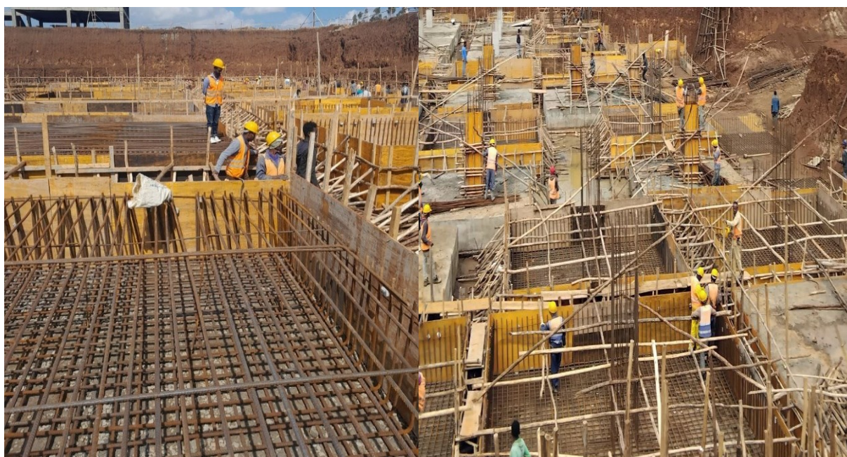
Figure 2.14 Rebar Placement for Isolated and Combined Footings Spaced by 5cm from the formwork.
