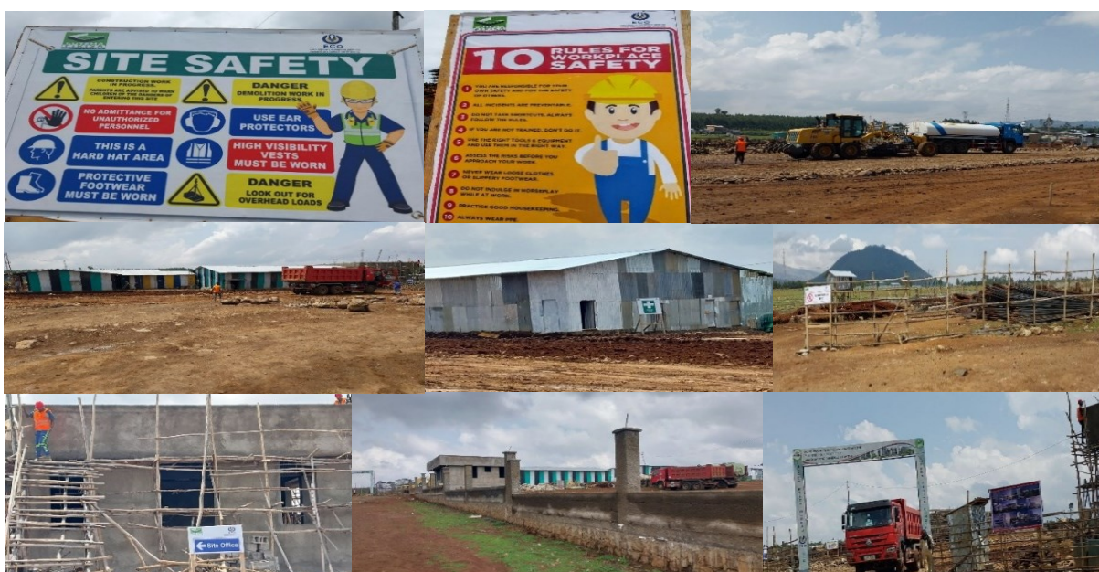
Figure 2.9 Site Layout before Mobilization, showing key facilities (i.e. Site Offices) and safety signage.
