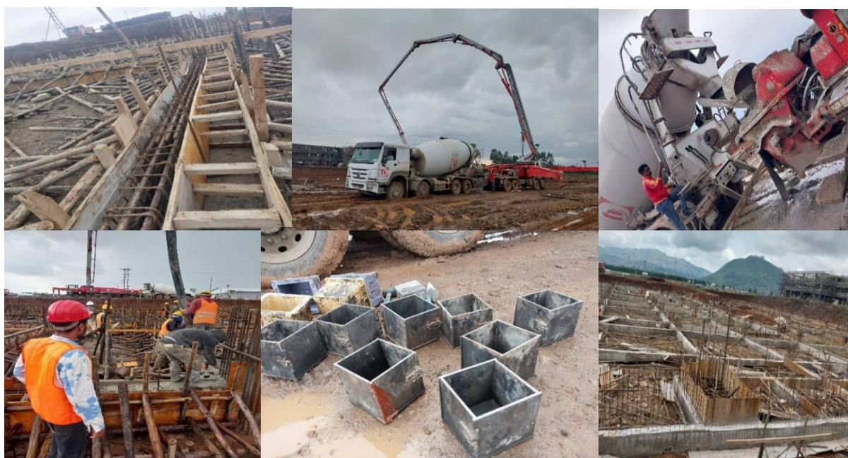
Figure 2.26 Basement Beam Concrete Placement, Vibration for Air Removal, Cube prepared for casting, and Formwork Removed beam.
