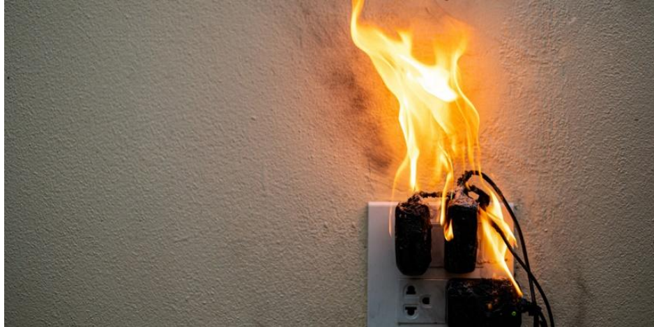
Figure 1 Burning of Electrical Wire Outlet due to Fault
