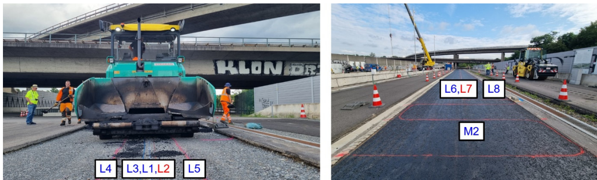
Figure 6: Views during installation and marking of the sensing cables (blue = strain, red = temperature), left: on unbound base course, right: in asphalt base course
