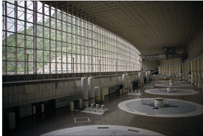
Figure 2.27: Sayano Shushenskaya's turbine hall before the accident, where turbine 2 (the turbine that failed) is in the foreground of the image a .
