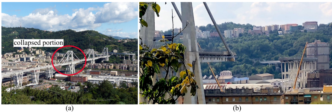
Figure 7.5: The Ponte Morandi bridge, showing the bridge: a) before the collapse b , and b) after the collapse c .
