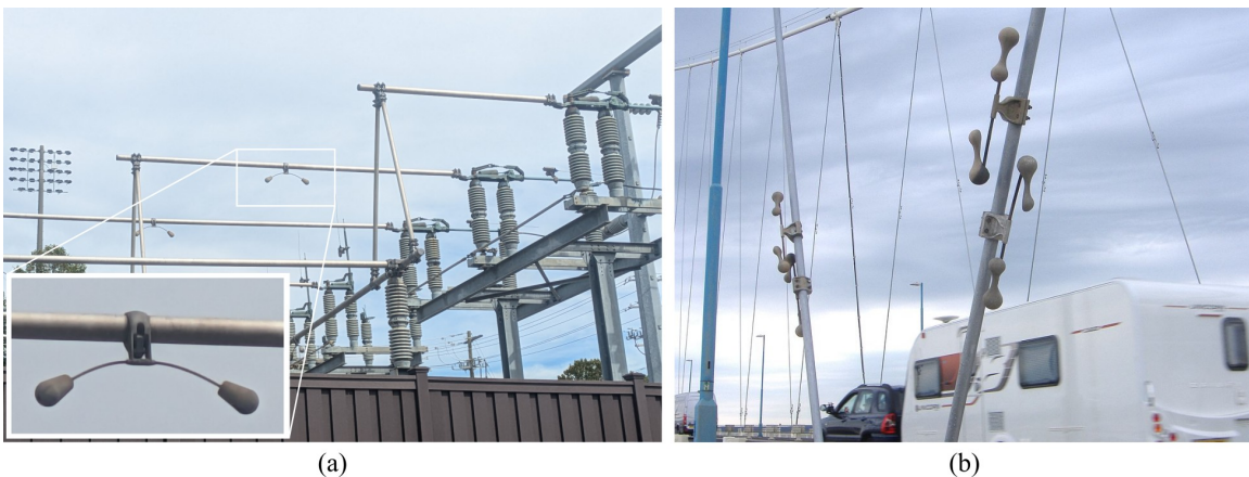
Figure 6.6: Vibration absorbers deployed on wind-excited cables showing: (a) a Stockbridge damper mounted on a rigid bus conductor in an electrical substation, and (b) a dogbone damper on a suspender cable of a suspension bridge a .
