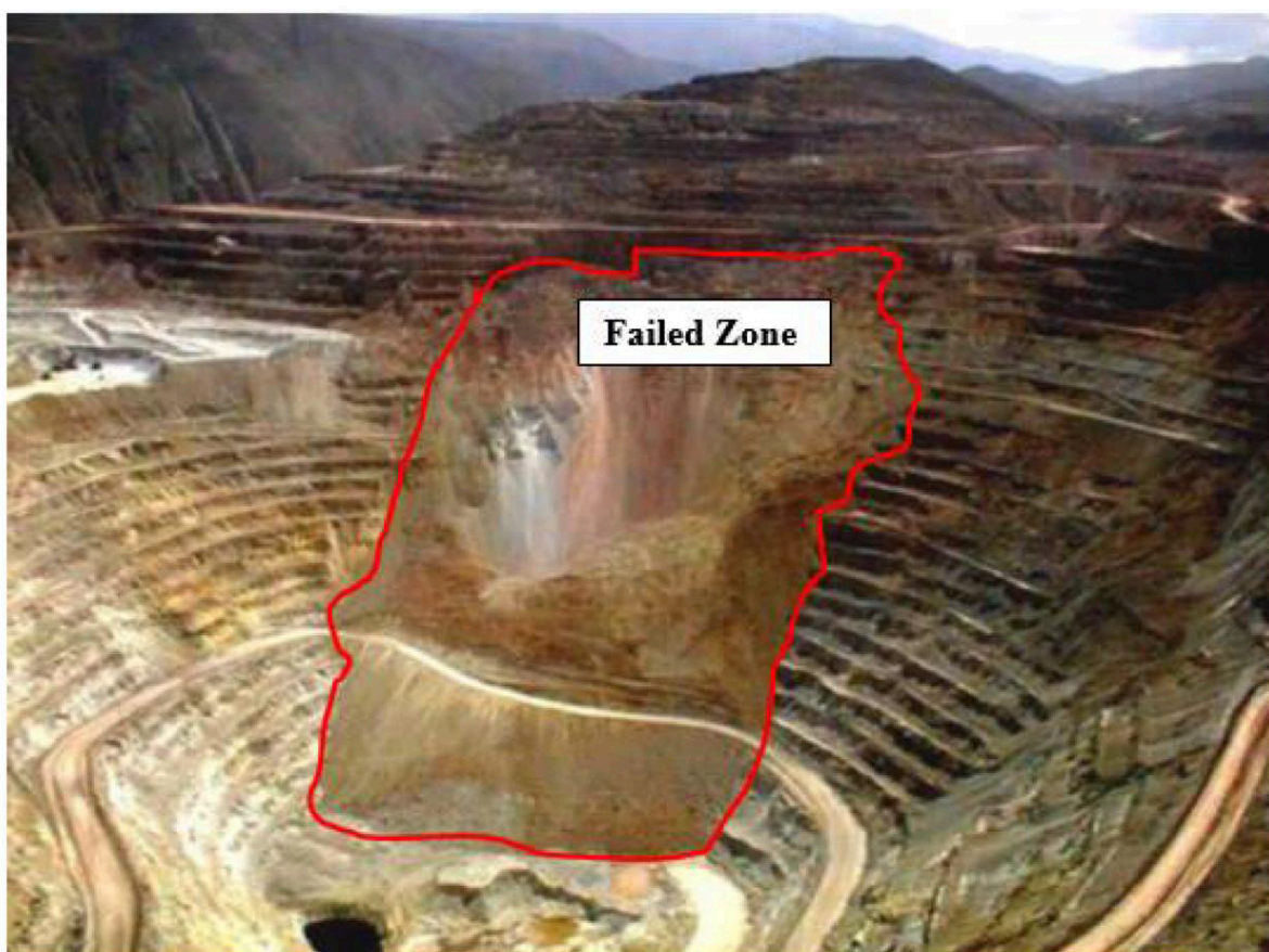
Fig. 1 A large-scale slope failure at a porphyry copper mine in South America
