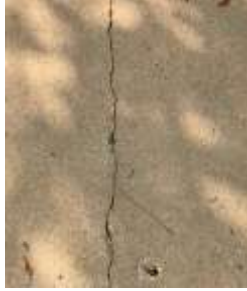
Figure 18. Original shadow crack image
