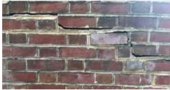
Figure 10. Original brick crack image
