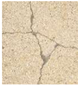
Figure 2. Original concrete crack image
