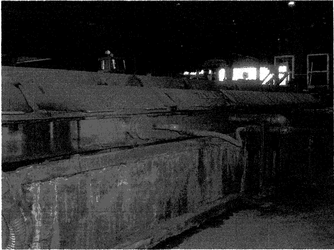
Figure 2-5: View of the Water Box
