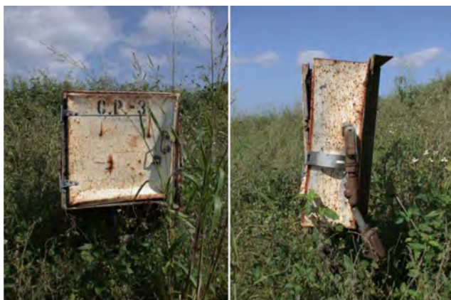
Figure-S 3.8 Damaged switch box, front face (left figure) and side view (right figure) [6].
