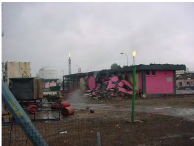
Figure-S 5.6 Panorama of the south side of Unit 40, electrical building, looking SE. Note the bent lamppost 38 E 25 and fence drawn inwards. (Private communication to GAC, 2004).
