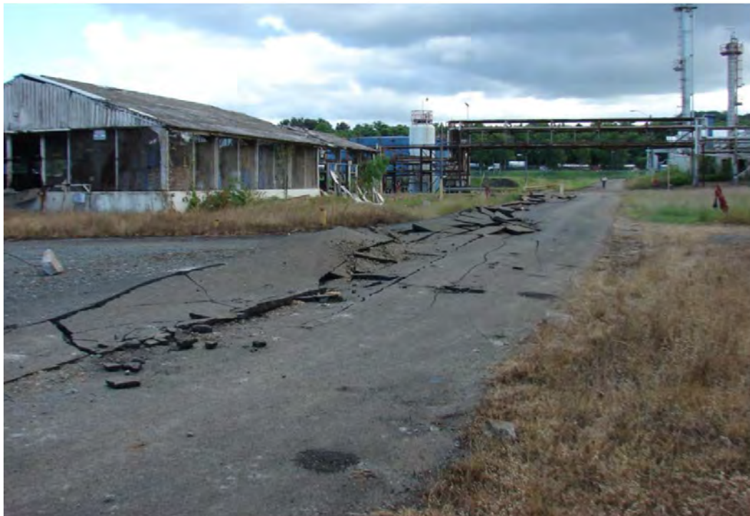
Figure-S 3.4 Damage to road above water culvert [6].
