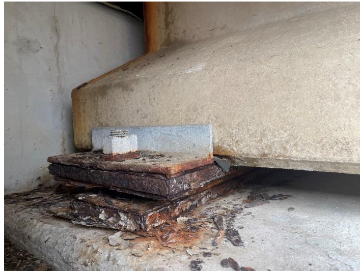
Figure 2. Field observations of corrosion-induced deterioration in elastomeric bridge bearing assembly with condition rating 3, showing severe rusting, section loss, and delamination of steel components due to prolonged exposure to moisture, water leakage, low clearance above water, and coastal and deicing salts.
