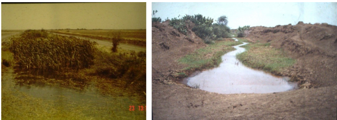
Plate (3) Sedimentation and Aquatic Weeds in Irrigation Canals (left) | Plate (4) Sedimentation Problem in Gezira Scheme Canalisation System (right)
