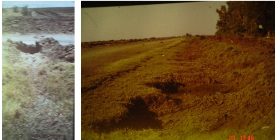
Plate (5) Irrigation difficulties in Gezira Scheme due to Sedimentation (left) | Plate (6) Poor Sediment Clearance of Irrigation Canal in Gezira Scheme (right)
