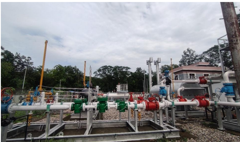
Figure: 1.15: 100 MW Power Plant (Temporary CMS), Shahjibazar.
