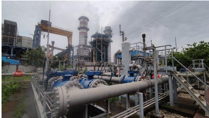
Figure 1.8: Bibiyana-3 Power Station- 400 MW
