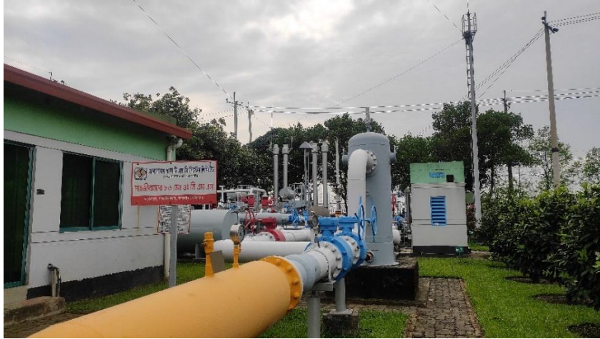
Figure 1.13: Shahjibazar Power Company Limited (86 MW)
