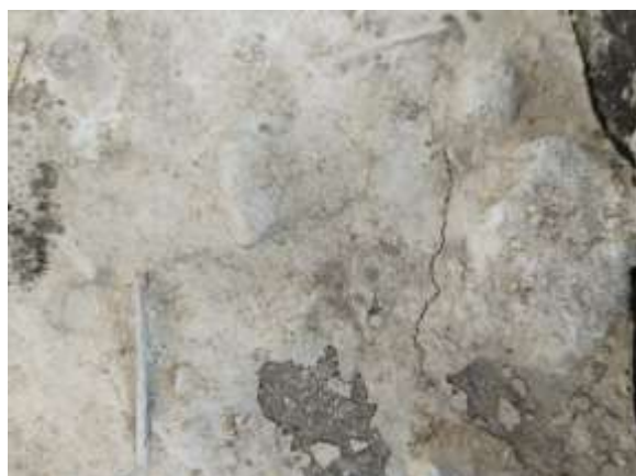
Figure 1 Cracks on specimen due to effect of shrinkage
